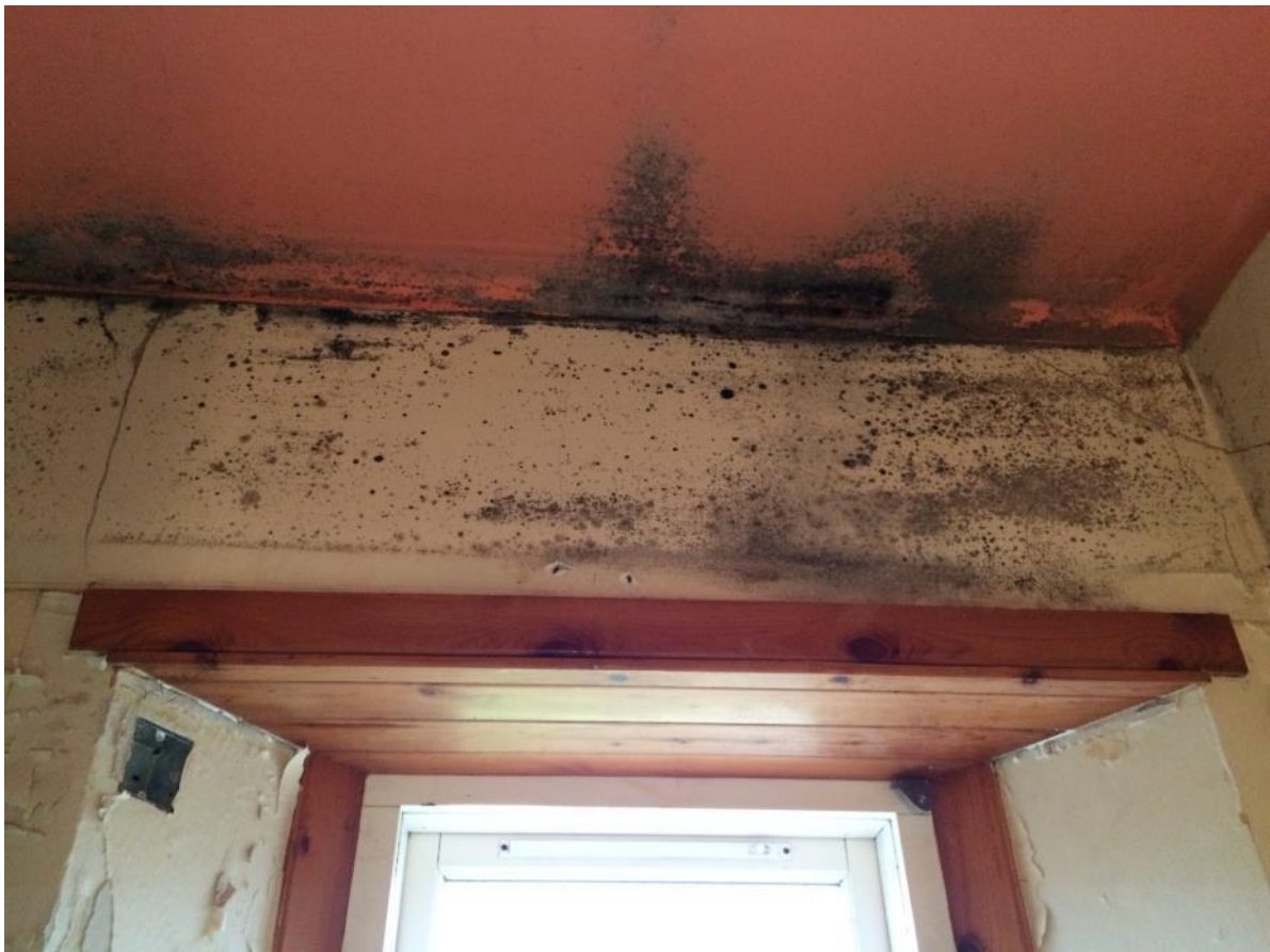
Figure 4: Mould uncovered in the bathroom following the removal of the lowered ceiling
